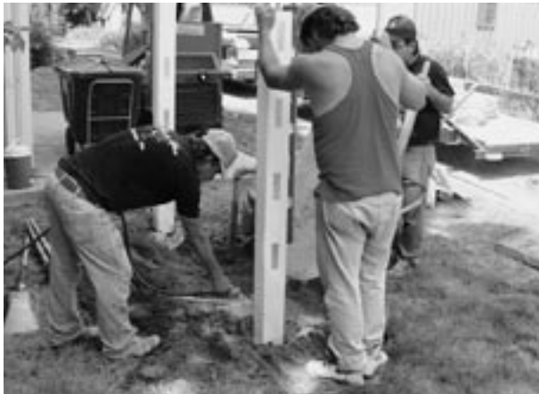
Holes dug, posts aligned and initially tamped in dry cement, water is being added to set the posts.
